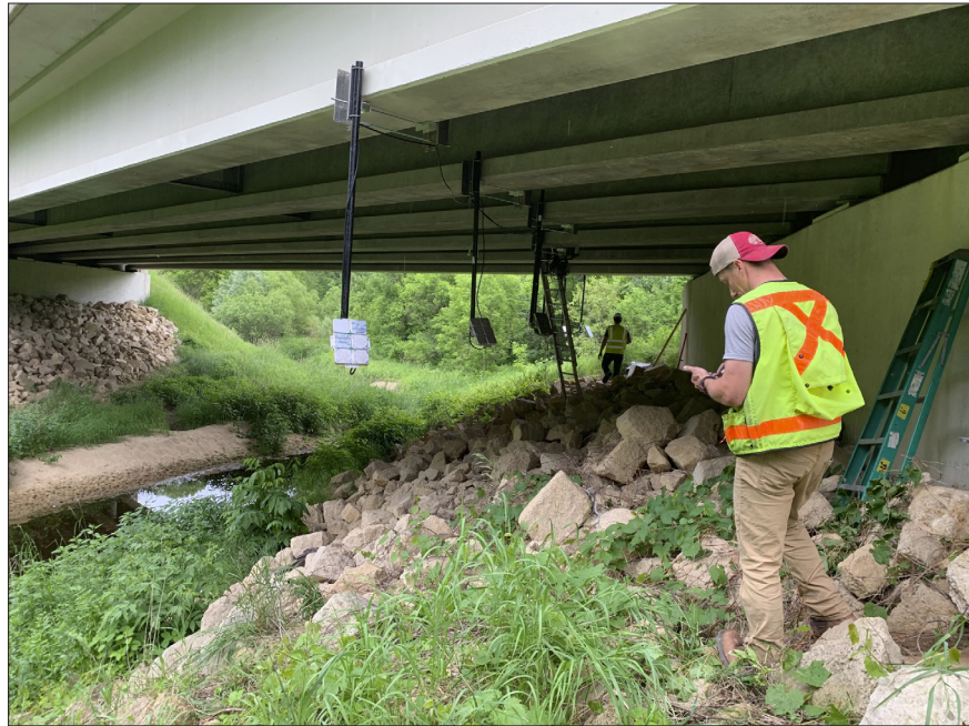
A Minnesota crew works with researchers to install ultrasonic acoustic bat deterrence devices under the deck of a bridge in Rushford Village, Minnesota.
